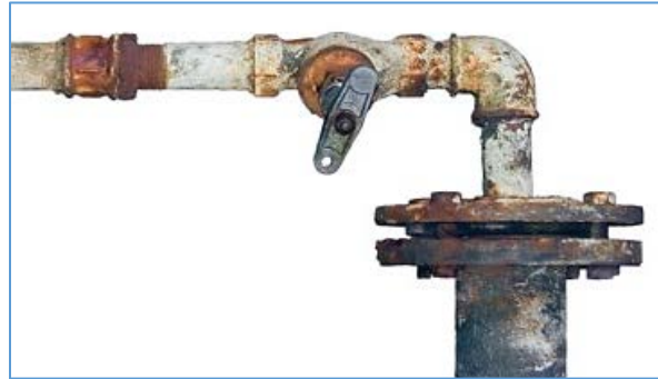
Figure 12: Corrosion from Dissimilar Metals
