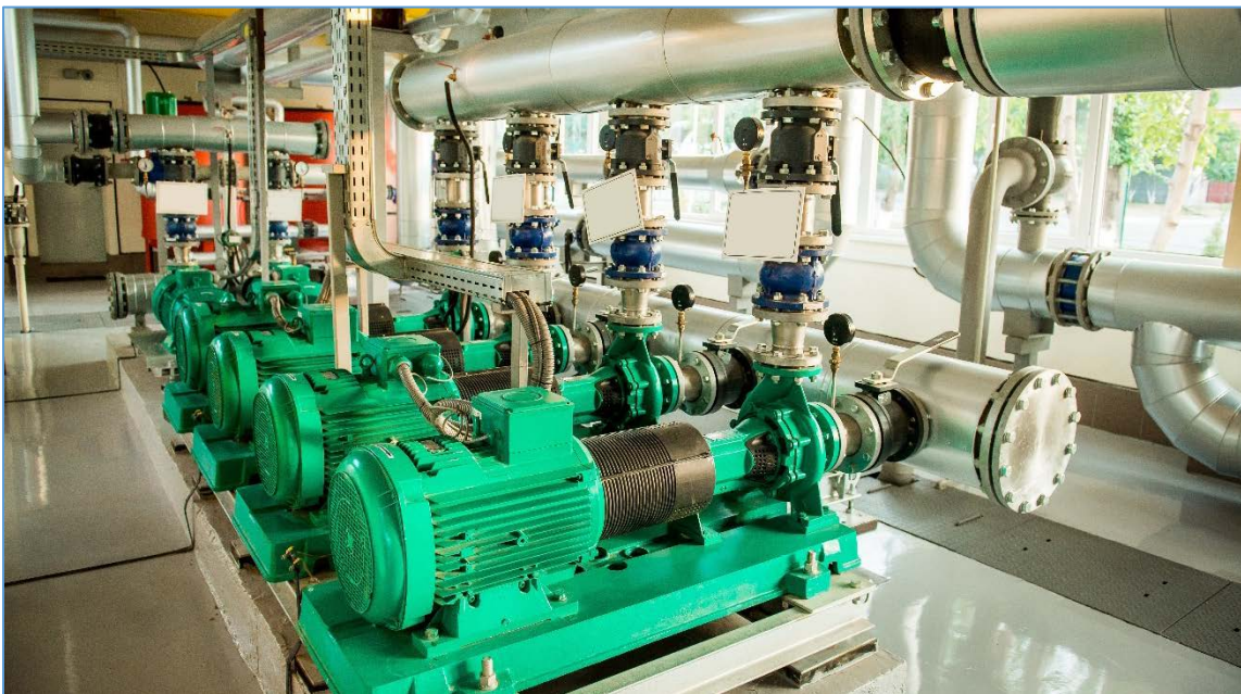
Figure 22: Modern Boiler Room
