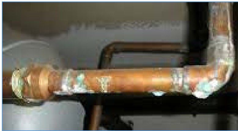
Figure 11: Corrosion from Carbonic Acid
